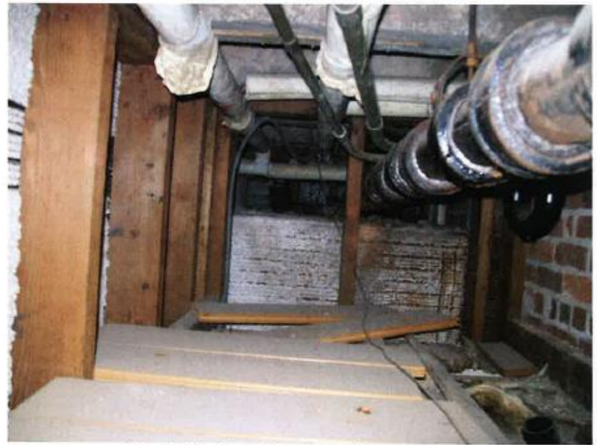
Pipe ACM inside wall cavity of 1 st floor boys' room
